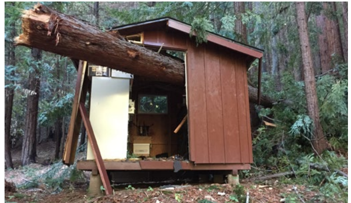
CBG's damaged storage building
